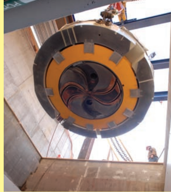
In 2008, part of the 220-ton particle accelerator was lowered into its underground home.
