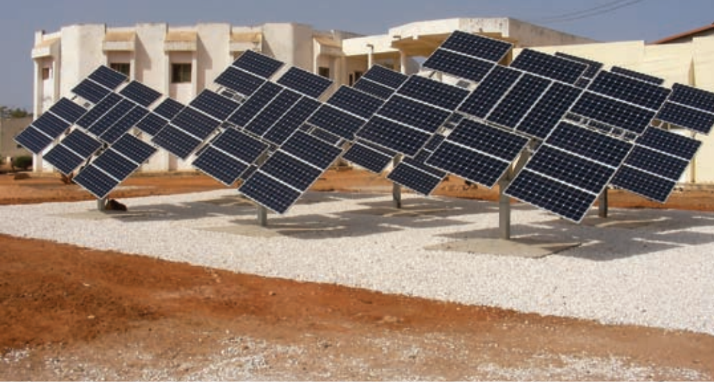
The solar panels are a good choice for a country that does not see rain for six months out of the year. Below, the OR staff can be more confident with a stable source of electricity.
